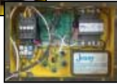
Electrical Junction Box
